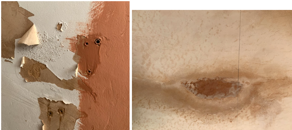
Figure 1. Examples of walls that need to be repaired prior application
